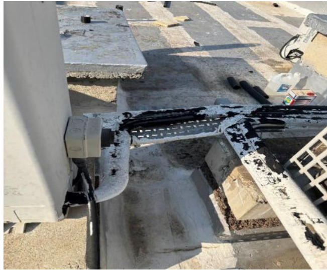
Figure 17: Piping wear and damages
