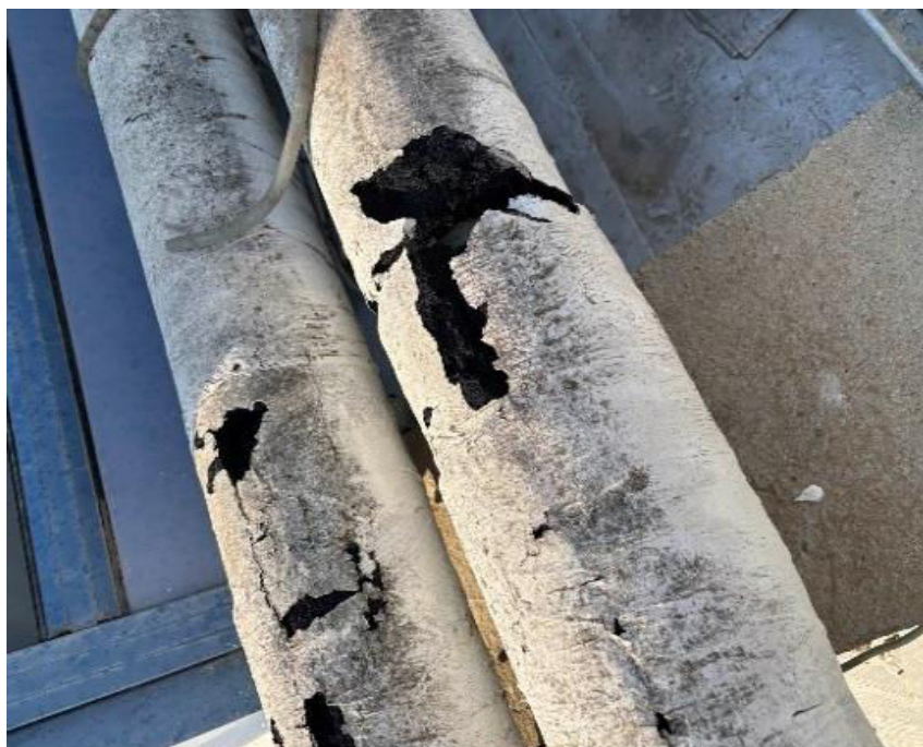
Figure 19: Piping wear and damages
