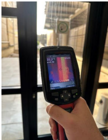
Figure 25: Eastern office window frame (14:05)
