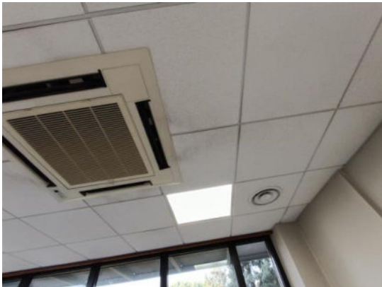
Figure 14: Leakage from the condensate pipe in the suspended ceiling
