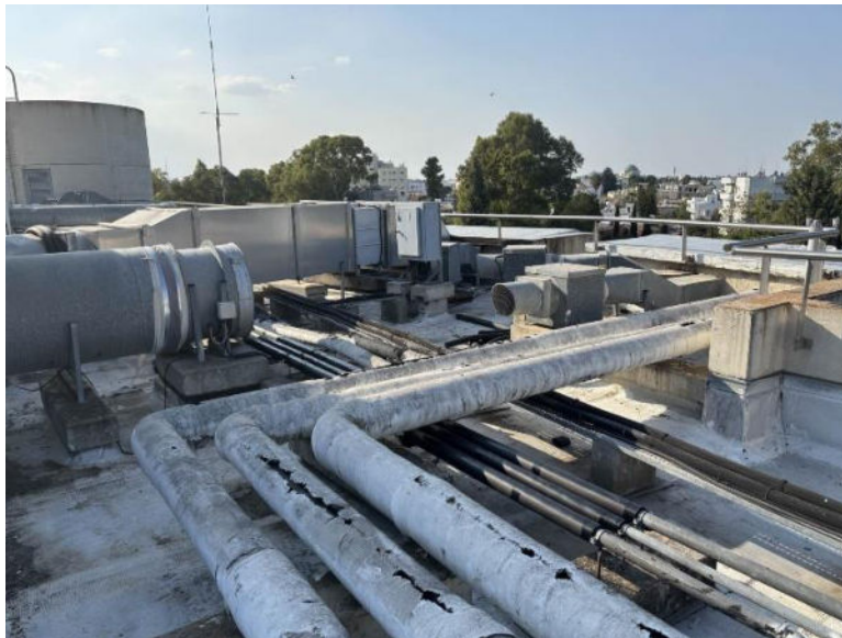
Figure 18: Piping wear and damages
