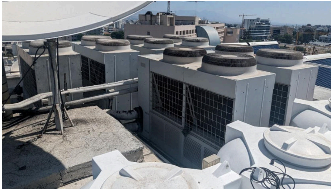
Image 4.4.1a. Six Chillers on the Roof of the Building
