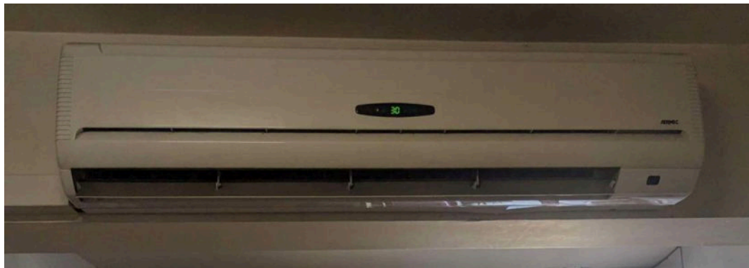
Image 4.4.1d. Split Unit of HVAC
