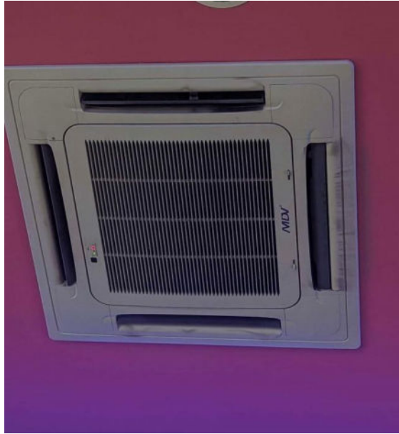
Image 4.4.1c. Cassettes of HVAC
