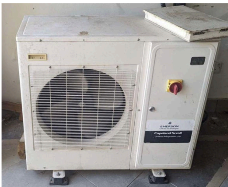
Image 4.4.4c. Compressor Cold Room
